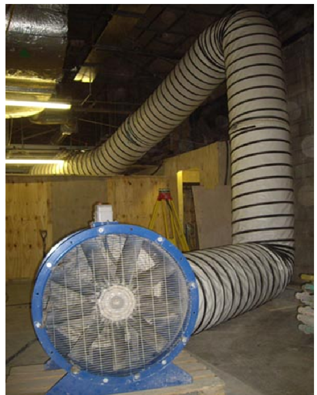
Temporary Ventilation System Blower plus Tubing
