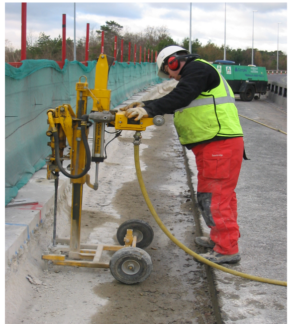
Works carried out on a bridge strengthening contract where client required dowel bars to be drilled into the existing concrete so new additional construction could be cast.
